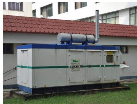
Diesel Generator Set
