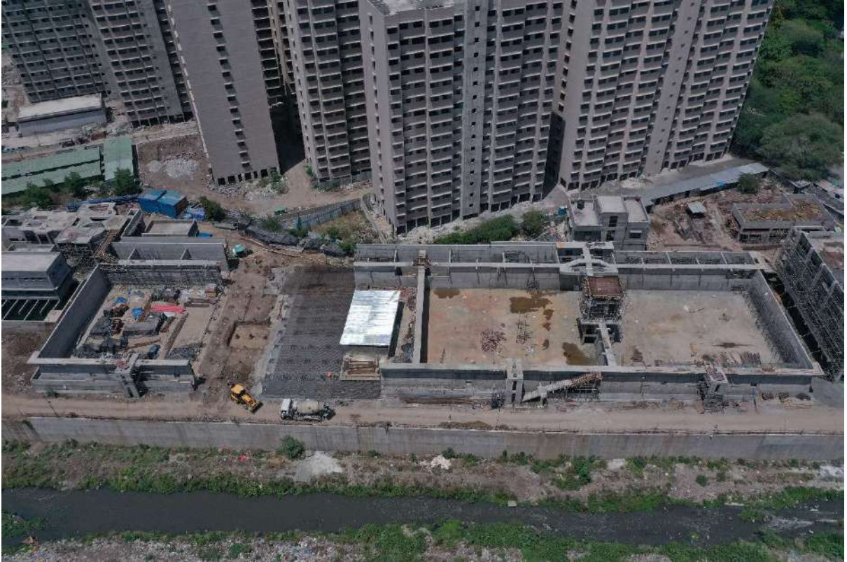
( Dhanori Sewage Treatment Plant – ૩૩ MLD )
